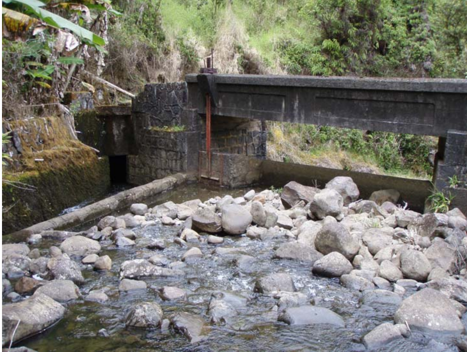
Figure 5-28. Photo of diversion on Honomanū Stream taken downstream of site 5. (6/30/2009; Tributary name: Honomanū (64009004); PBN: In005p-007-063009; Surveyor: Nishiura, L.; SBN: In005d-063009; Lat. (DD): 20.83271, Long. (DD): -156.18056).
