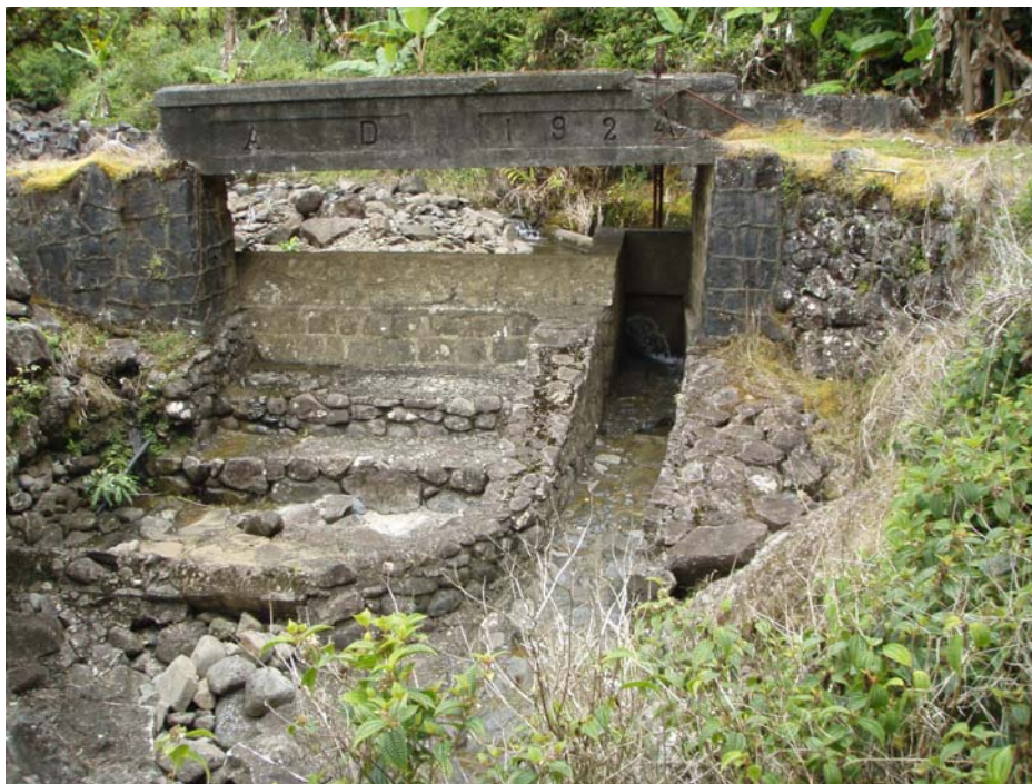
Figure 5-26. Photo of a bridge crossing. (6/30/2009; Tributary name: Honomanū (64009004); PBN: dk004p-004-063009; Surveyor: Kuamo‘o, D.; SBN: dk001d-063009; Lat. (DD): 20.83271, Long. (DD): -156.18056).
